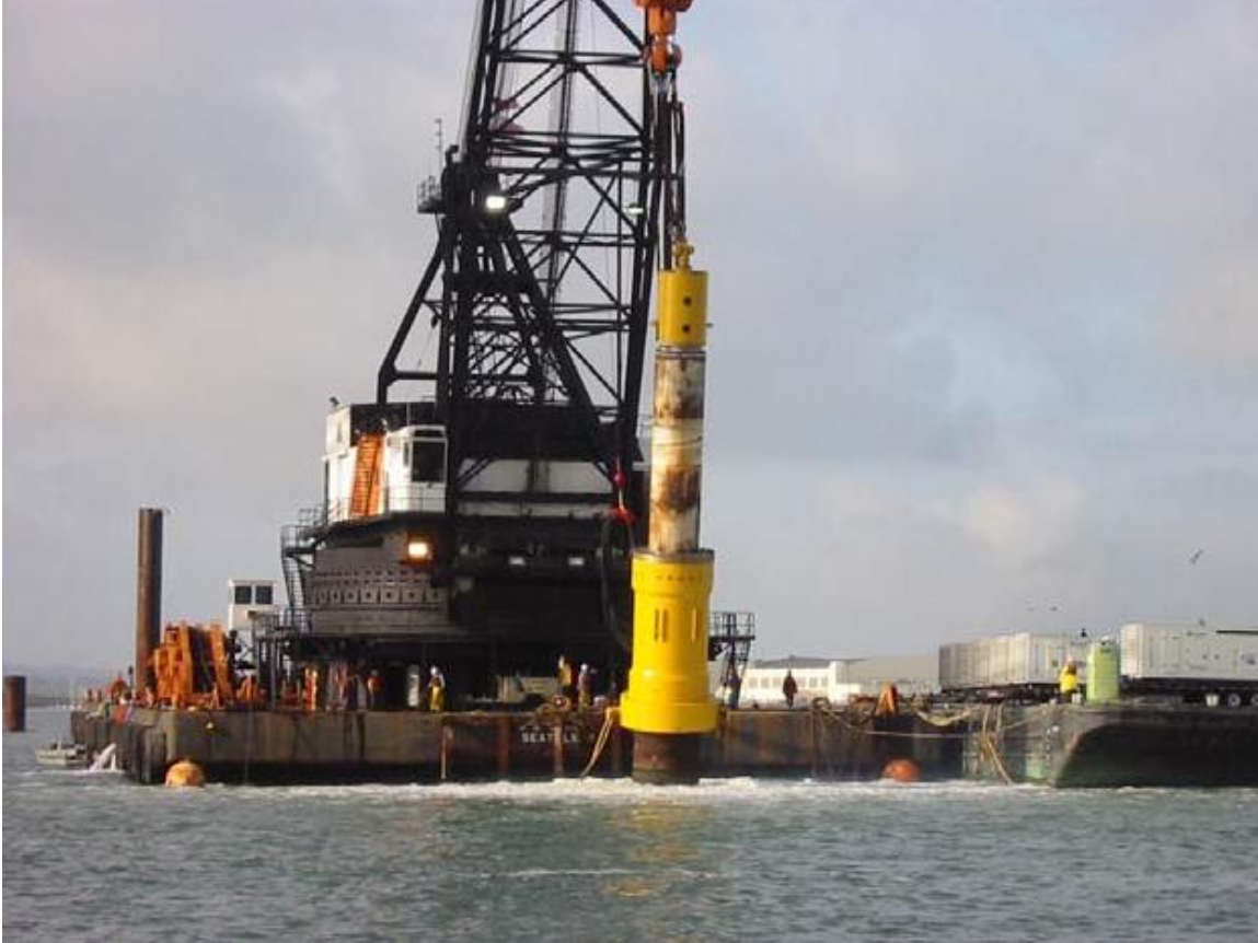
Figure 1: Impact pile driving of a 30"-diameter, partially submerged CISS pile at the Friday Harbor Ferry Terminal on San Juan Island (Carlson and Weiland, 2007)
